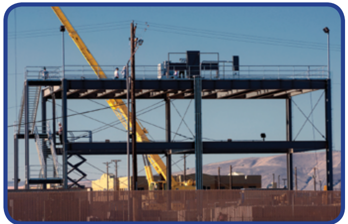
Columbia Energy is erecting a fully integrated test center to aid Department of Energy contractors.
