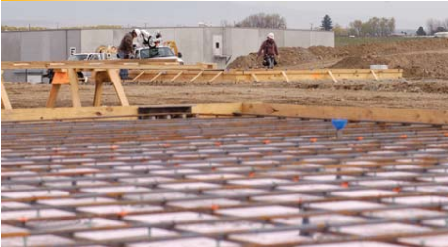
Construction of the Mercer Estates winery is under way with an expected completion date in September.
